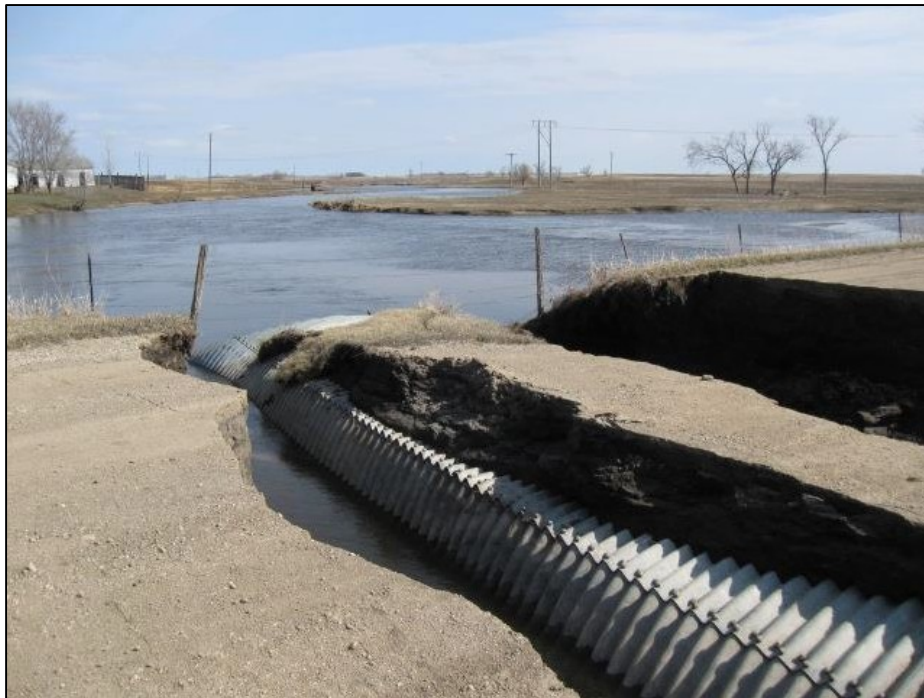
Example of a Category C claim with road embankment washed out completely but culvert may be salvaged. (credit: North Dakota Department of Emergency Services)
