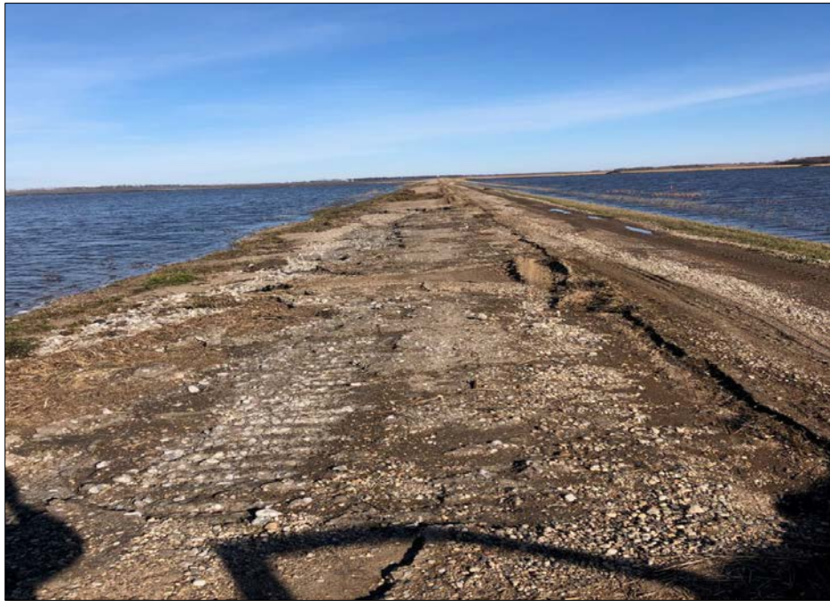
Example of a road that was completely submerged in water for an extended time. Debris needs to be cleaned up and re-graveled. (credit: North Dakota Department of Emergency Services)
