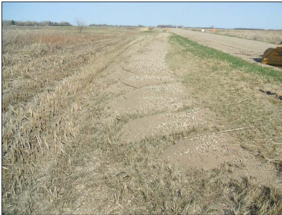
Example of gravel surfacing washed away, take pictures for site documentation before grass grows through it. (credit: North Dakota Department of Emergency Services)
