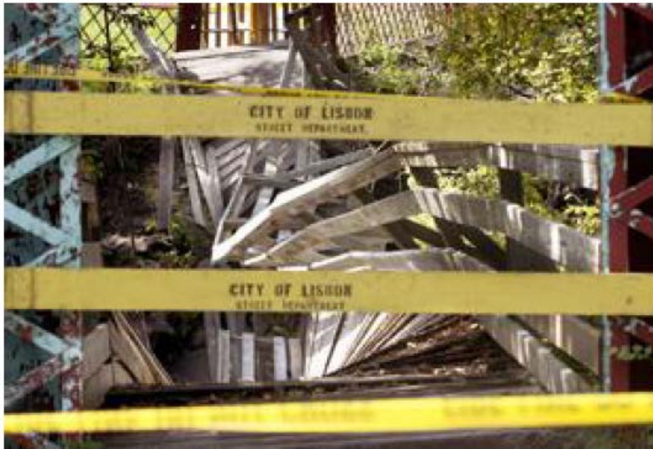
A wooden walking bridge over the Sheyenne River in Lisbon, N.D., is a twisted mess Thursday, Sept. 25, 2008, after it collapsed Wednesday, injuring five construction workers who were taking a break on the bridge. Authorities said two of the men were treated and released and three others were taken to Fargo hospitals. No names or conditions were immediately available. (AP Photo/The Forum, Dave Wallis)
