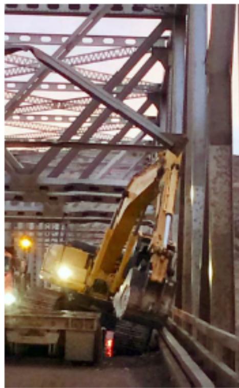
The most recent hit on the Long X Bridge near Watford City came Nov. 22 when an excavator on a trailer hit the bridge's overhead framing. Special to The Forum
