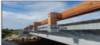
A St. Louis County composite timber and steel bridge features wooden railings.
