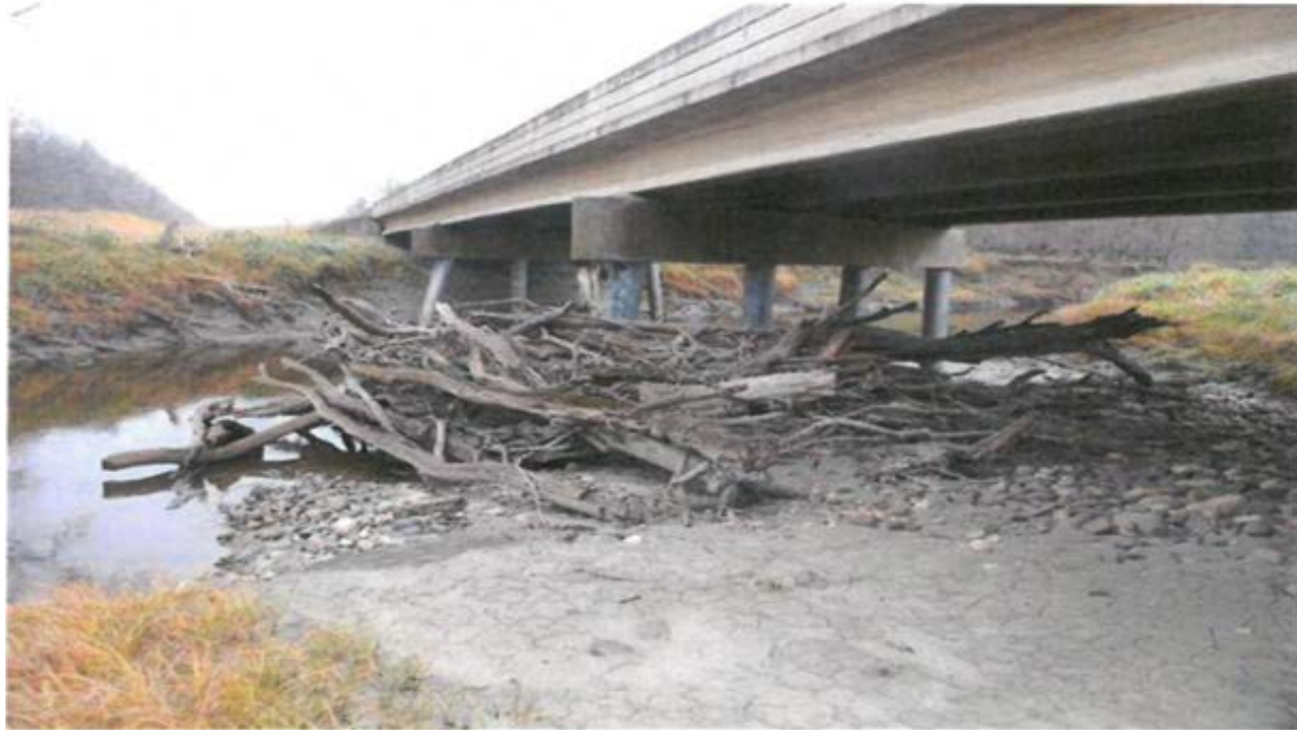
Photo 3 - 10-31-16 Large pile of debris hung up on center pier
