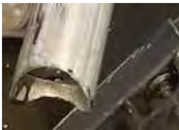
Divoted pipe at outflow point
