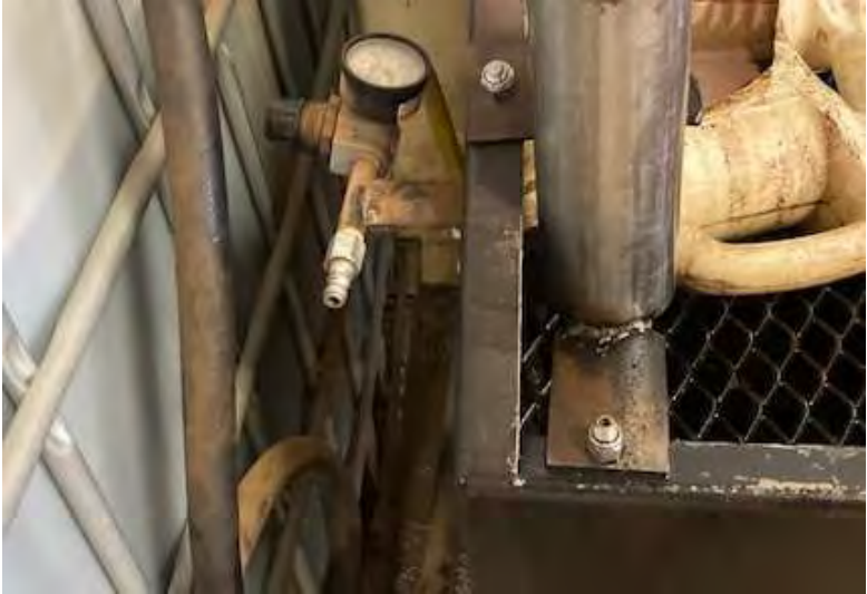
Air compressor connection for air pump
