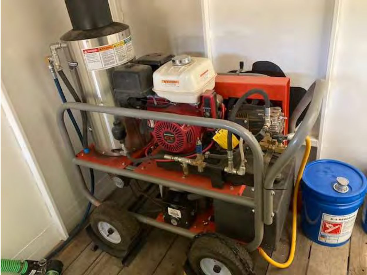
Power washer/water heater unit
