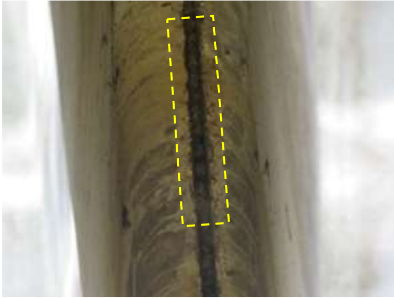
Stains from Minor Corrosion of Steel Plates
